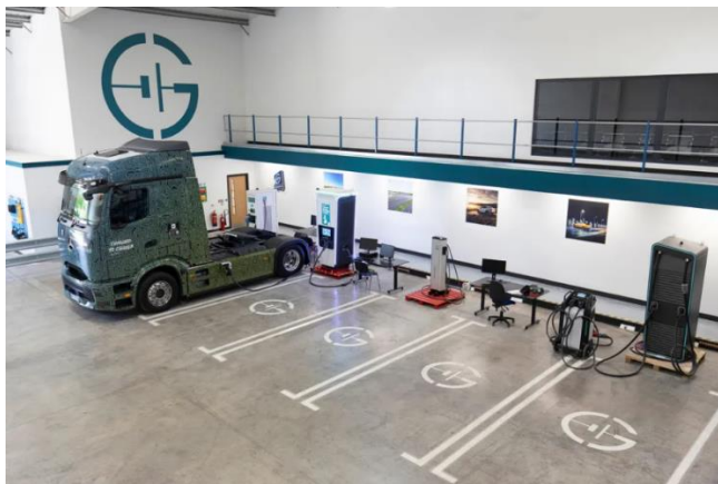
Figure 4 - GRIDSERVE's EV charging test lab
